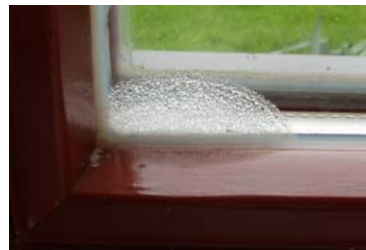
Picture 6.2 – water attack defect
