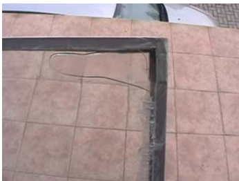
Picture 6.1 – Water attack defect
